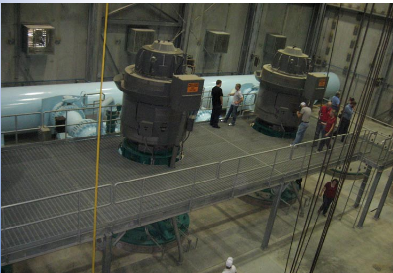
Inside the pumping facility at the East Fork Raw Water Supply Project.
