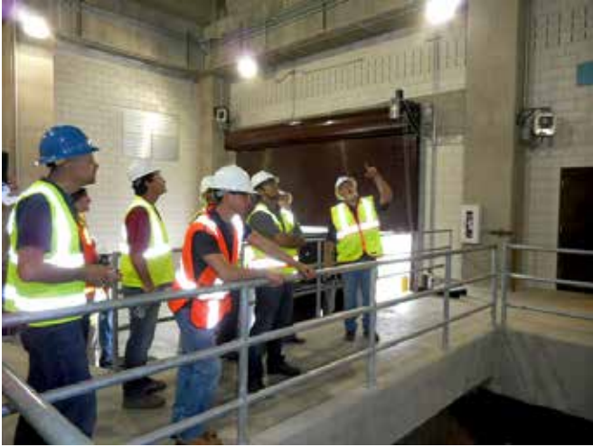
YPs listening to Mr. Mark Reed (Trinity Watershed Management) explaining the construction of the Pump Station.
